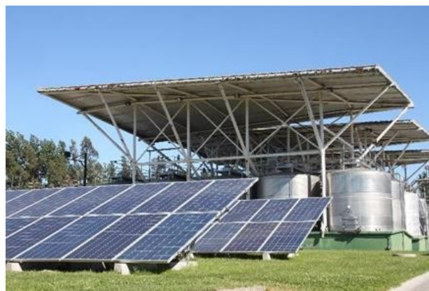
Photo 9. Solar panels installed in the Miguel Torres winery in Curico, Chile, photo J. Rochard.
